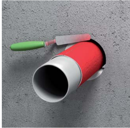
2. Ensure smoke tight seal of the annular hole (e.g. with Pacifyre® FPM Fire Protection Mortar or Tangit FP 430 Fire Protection Acrylic Sealant)
