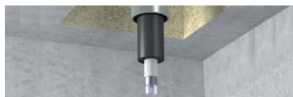
Multi-layer pipes with insulation
